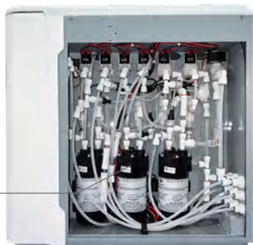
Two-stage booster pump
